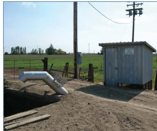
Typical Pumping Plant
